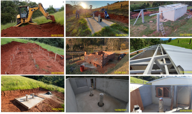
FIGURE 5. Observatory build photos and milestones. The leftmost column shows the first build phase in early 2020 (terrain, dual concrete piers and observing slab); the center column, the first part of the second phase in Sep. 2021 (walls and heavy civil construction); the right column shows the second part of this phase in Dec. 2021 - early 2022 (roof assembly and finishing).
